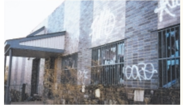
Before, the abandoned building was located in a distressed area of Philadelphia.
